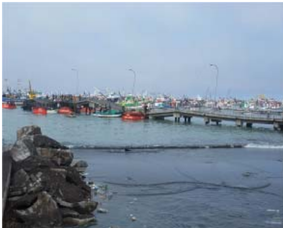
Photo 18 Damaged pier in Coronel
