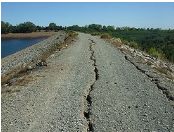
Photo 9 Longitudinal cracks at the crest of Coihueco Dam
