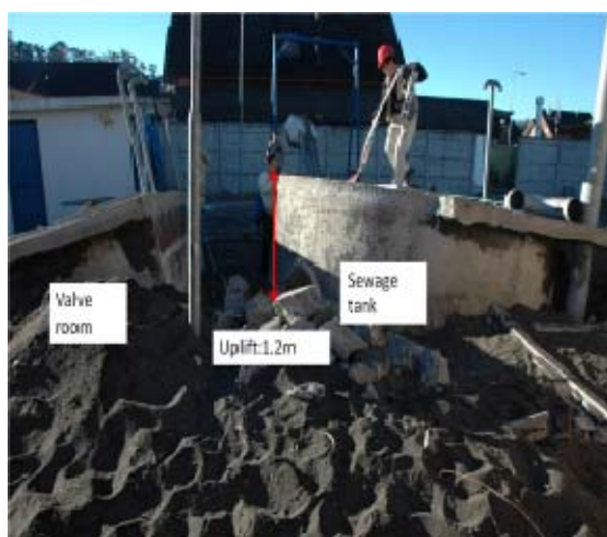
Photo 3 Uplift of buried sewage tank in San Pedro de la Valle
