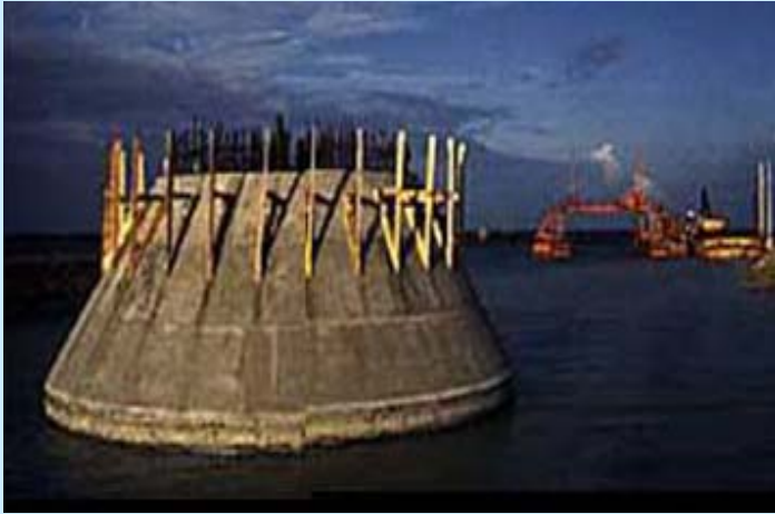
Gravity base foundation being floated out to Tunoe Knob Photograph © 1996 by Flemming Hagensen
