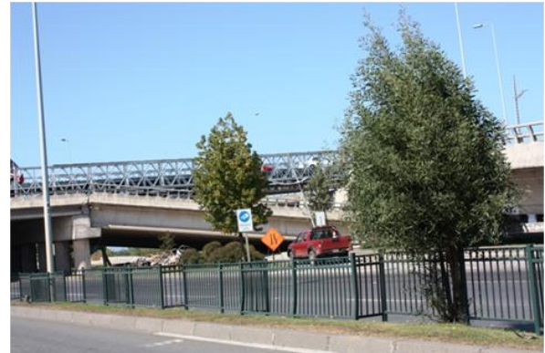
Figure 3. Provisional metal bridge over collapsed section of bridge over Bío Bío river, Concepción.
