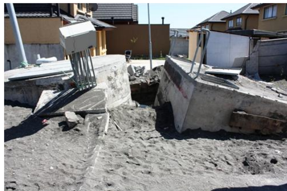
Figure 15. Flotation of boxes of a treatment plant in San Pedro La Paz.
