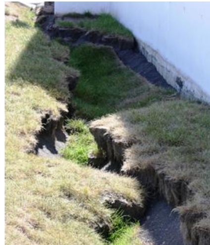
Figure 14. Cracking parallel to the school's constructions, caused by liquefaction. San Pedro La Paz.
