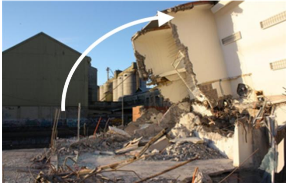
Figure 23. Final tension failure of the front portion of the ground floor, which determined the building's overturn and collapse.
