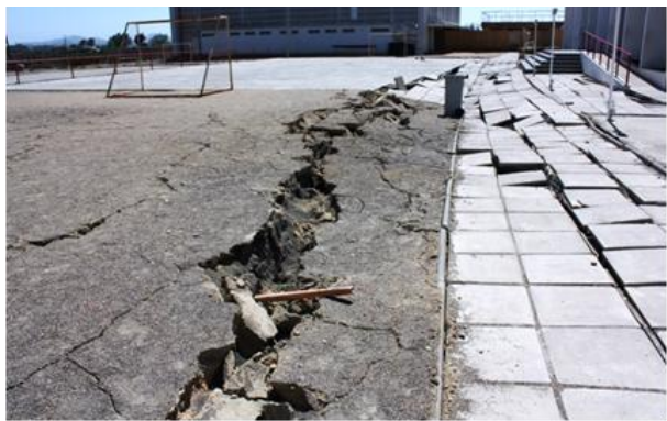
Figure 13. Liquefaction at a school's patio in San Pedro La Paz.
