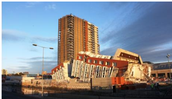
Figure 1. Overturned “Alto Río” building in Concepción.
