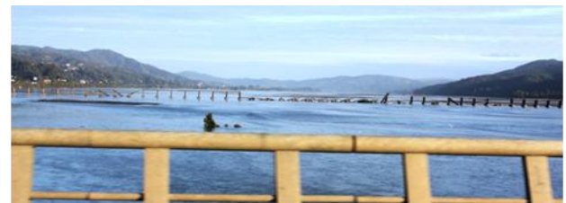
Figure 4. Multiple collapsed panels of “old” bridge over Bío Bío river.
