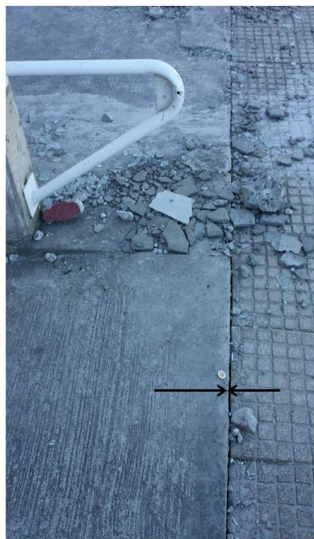
Figure 24. Lateral displacement of the foundation box of only 6 mm.
