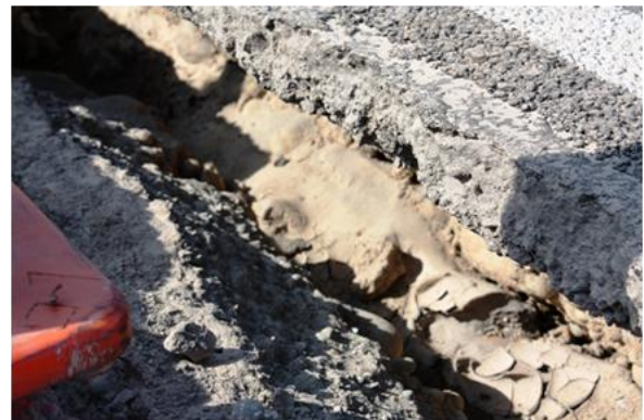
Figure 10. Liquefaction on road 5 South, Santiago-Concepción.
