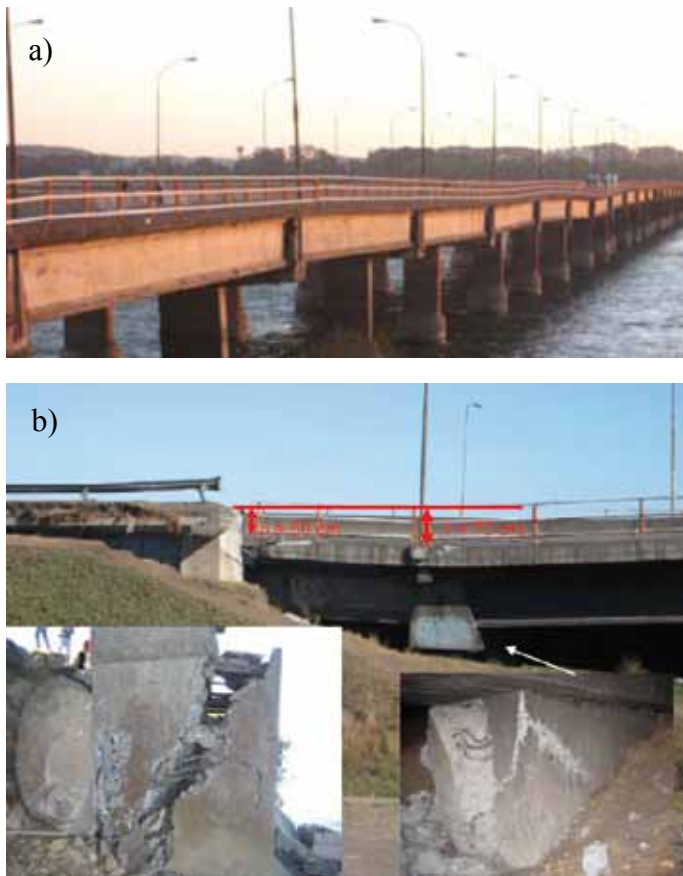
Figure 11: Juan Pablo II Bridge showing a) unevenness due to pier differential settlements and b) shear failure in reinforced concrete piers
