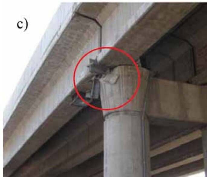
Figure 8: Damage in bridges of type 3 configuration: a) shear key failure detail b) and c) lateral displacement of girders in Vespucio Norte at Independencia.
