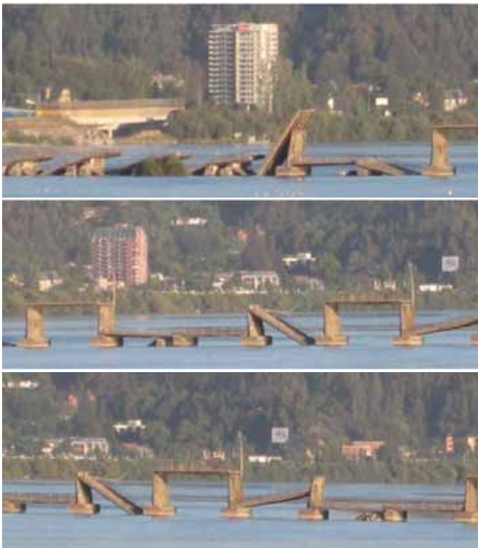
Figure 12: Sections collapsed of the Bío Bío Old Bridge
