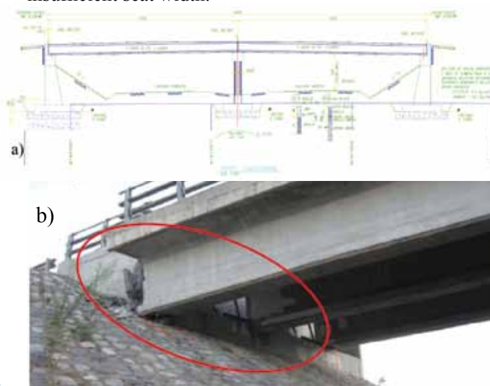
Figure 6: Damage in Las Mercedes underpass, bypass Rancagua, route 5.
