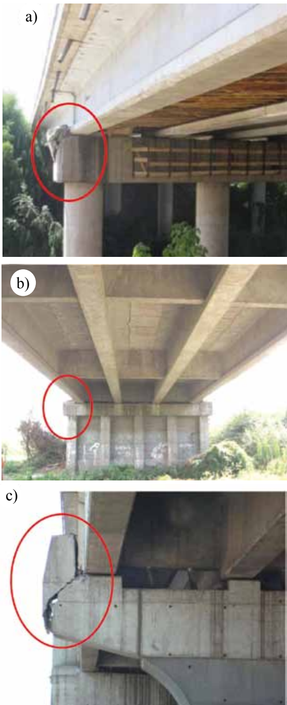
Figure 3: Damage in bridges of type 1 configuration: a) Costanera Norte, b) Lollole and c) Vespucio Norte at Independencia
