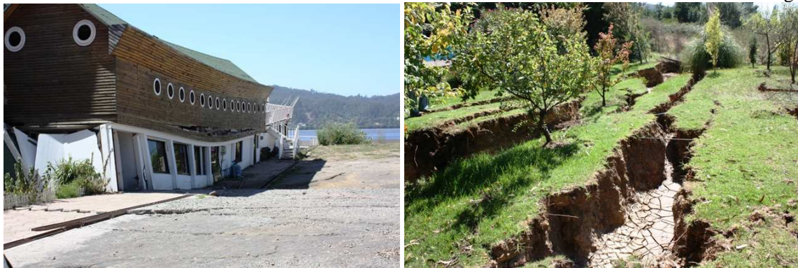
Figure 6: Damage in a restaurant, garden and piping due to lateral spreading along Santa Juana road
