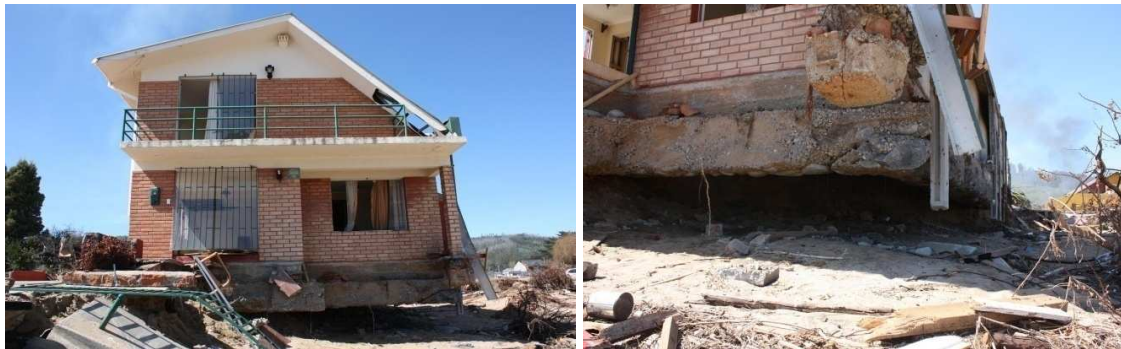
Figure 9: A house in Dichato with foundation exposed due to scour by tsunami
